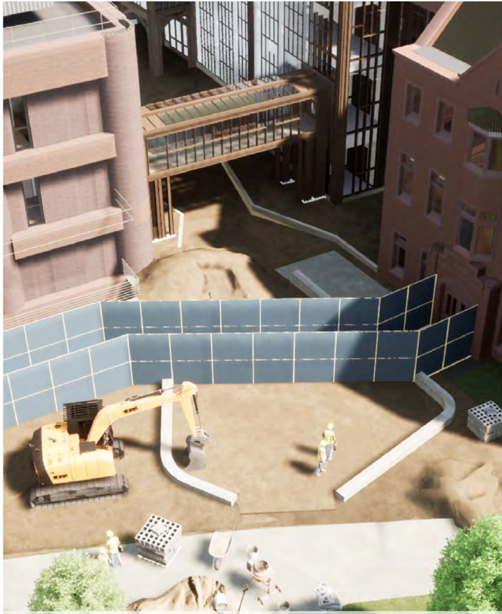
Yale Peabody Museum of Natural History Additions and Renovations [ Logistics Plan ] - SITE LAYOUT AND ACCESS
